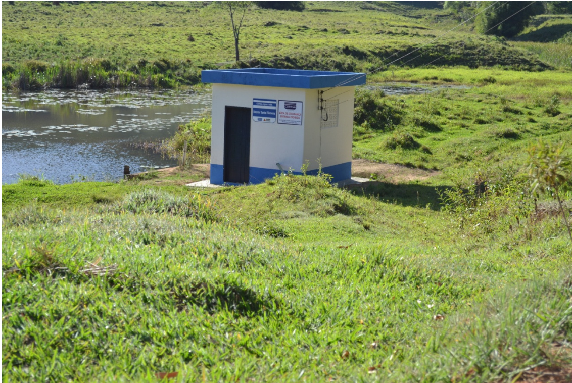
Figura 11: Booster Santa Filomena. UTM – 708498/7678200.
